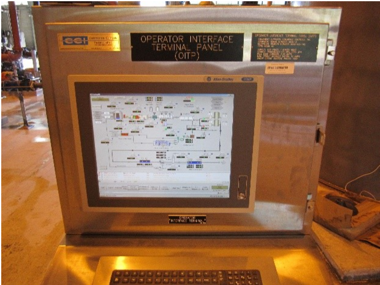
Figure 4-6. SCADA system at a Superfund site.
