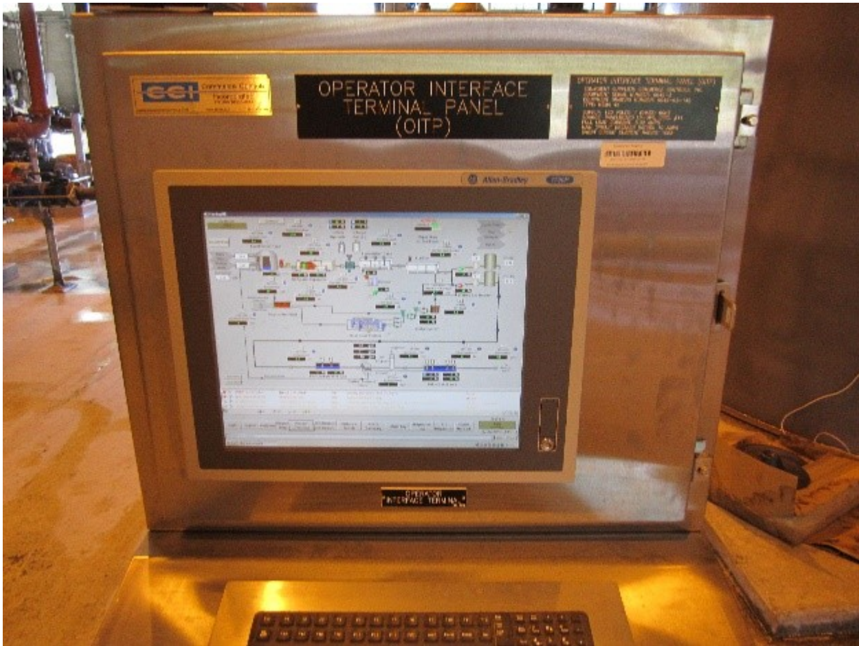
Figure 4-6. SCADA system at a Superfund site.
